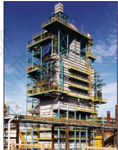
Ethylene Cracker Unit
